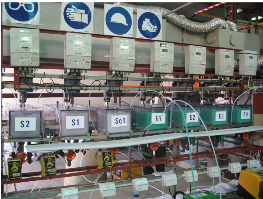
Figure 2. Rear view of pilot plant, showing mixing boxes, dosing lines, pH controllers, and pumps.
