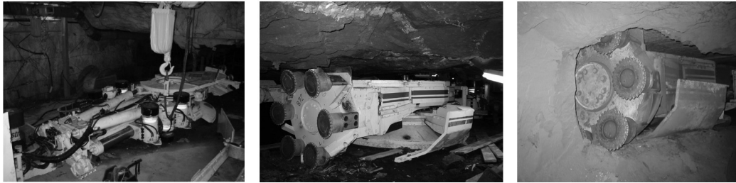
Figure 6. Assembly of the ARM 1100, launching the machine and cutting into the raise
