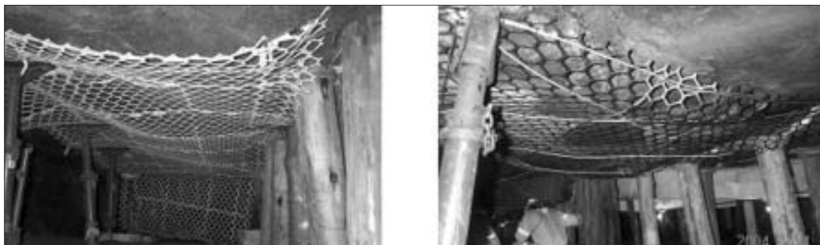
Figure 6. Photographs of the current types of safety net installations at Impala Platinum Mine
