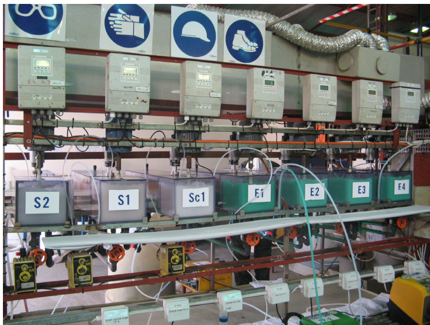
Figure 2. Rear view of pilot plant, showing mixing boxes, dosing lines, pH controllers, and pumps.
