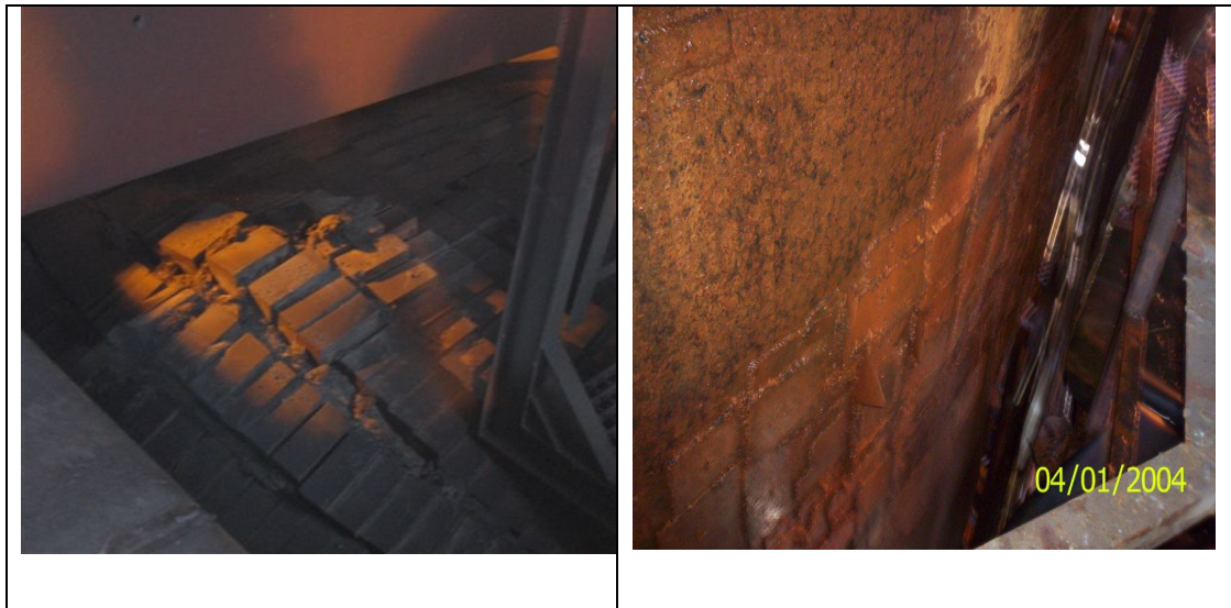
Figure 3. Reaction shaft roof damage
